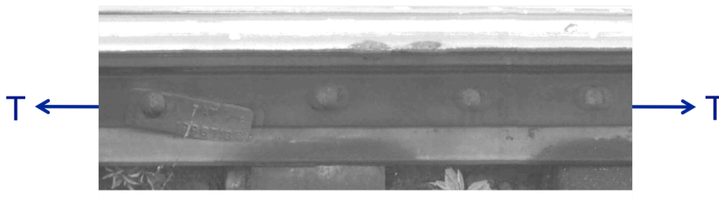
A: Original Image Switch Point Bolts
